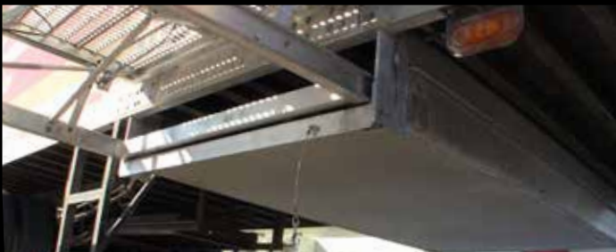
Elevated Platform protected within a fully closed enclosure box
